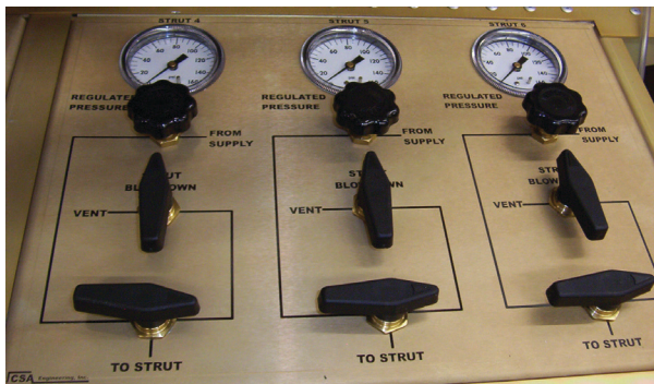
Figure 7: Strut control panel.
